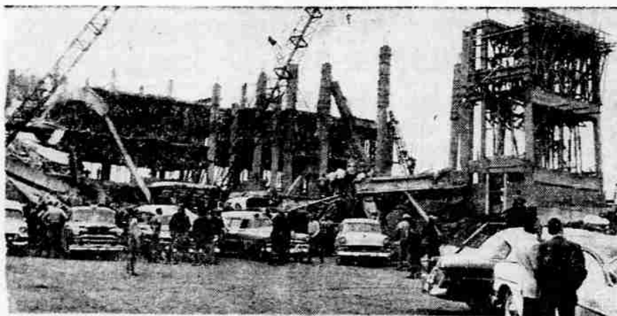
MOVING TONS OF DEBRIS, cranes probe wreckage of building under construction at Jackson, Mich., in which 10 workmen lost lives when fourth floor collapsed. (International)
