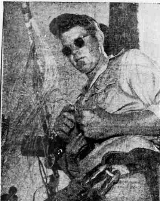
CABLE SPLICING —The job of cable splicing is considered a delicate one. Here Pacific Telephone Splicer Gene Rosencrans connects tiny copper wires in cable strung from poles along Hillcrest rd.
