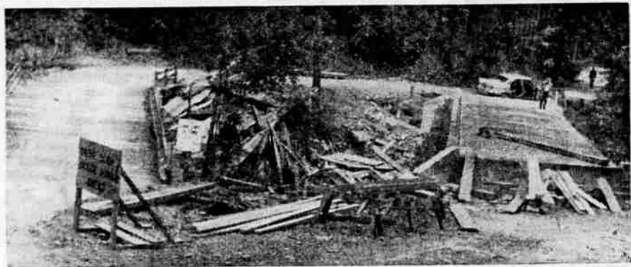
DETOUR IN USE —County road crews constructed a wood detour bridge (left) before blasting out remainder of the log bridge built approximately 14 years ago by soldiers stationed at Camp White. The new bridge could
