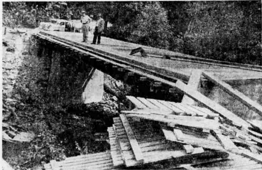
CONSTRUCTION STARTED —County Judge Rodney Keating, left, and Commissioner L. G. (Shy) Morthland stand on the partially completed Carberry Creek bridge being constructed in southwestern Jackson county near Steamboat. Concrete piers were built by
