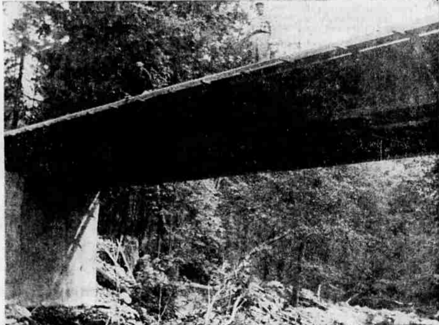
READY FOR RAILING —West Coast Steel company, Portland, will install railing and complete other steel work on Carberry Creek bridge sometime this week. County crews have done most of the concrete work. The bridge has three steel spans measuring 63
