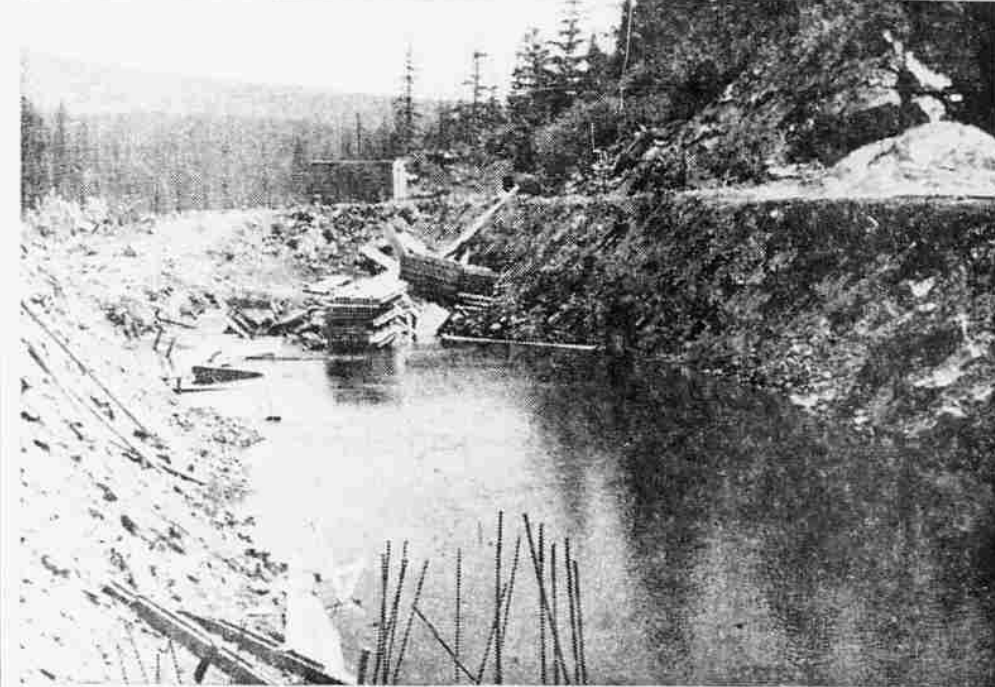
SPILLWAY SITE —A concrete-lined side channel on the left abutment at Fish lake will provide an adequate spillway. Construction will start on the 90-foot long spillway as soon as the irrigation season is finished. Head of the structure will be at left center in above picture.
