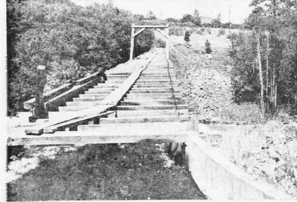
LAKE CREEK SIPHON —A 60-inch precast concrete siphon 345 feet long will replace this 460-foot metal flume at Lake Creek. Loose rock at right of structure is where the new siphon will be constructed once water has stopped flowing later this year.
