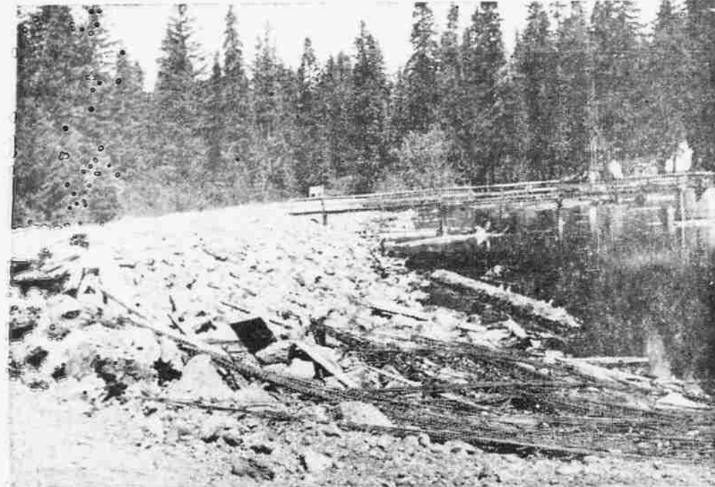
RIP-RAP WORK —New rip-rap was placed along the face of Fish lake dam earlier this year to reinforce the face of the dam. Rock was taken from the site of the new spillway, which will be constructed to the right of construction metal in foreground.
