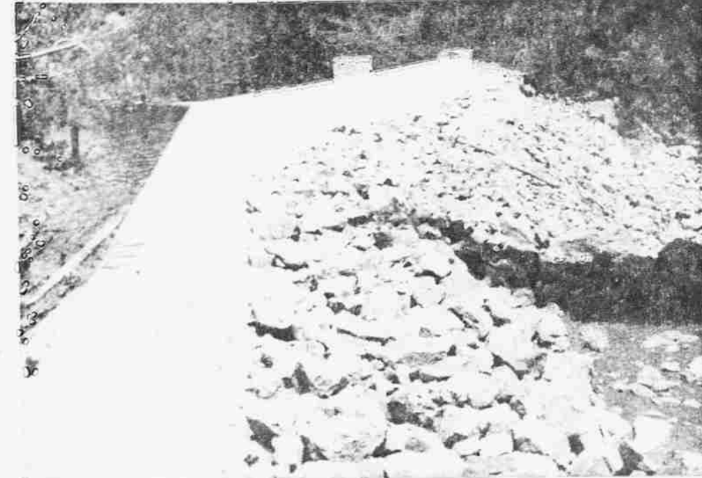
PARAPET WALL —The 175-foot long 3 1/2-foot high parapet wall along the crest of Fourmile lake dam, one of two rehabilitation structures, is shown above. The wall was constructed to prevent water, in high winds, from washing over the top of the dam.
