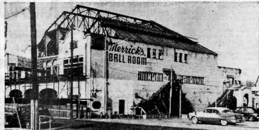
GOING, GOING... — Merrick's building—also known over the years as the "Natorium" or "Nat," and also the ballroom—one of Medford's landmarks, virtually vanished last week, as wrecking crews neared completion of the demolition job. The picture at the left shows how the building appeared just as the tearing-down job was started several weeks ago. The view at the right shows how it appeared last week, with only a few girders and one or two smaller walls and archways remaining.
