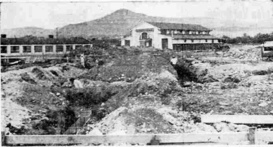
EXCAVATION UNDER WAY —Excavation is under way for the foundation of the National Guard armory at the old county fairgrounds site on Highway 99. The building will replace the old armory on North Bartlett
