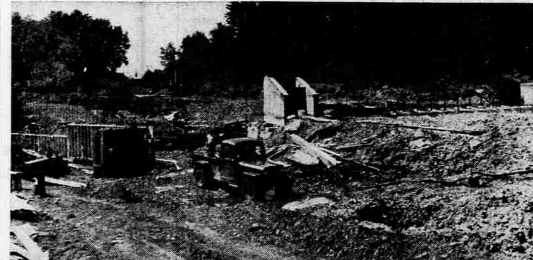
REPAIR FLOOD DAMAGE—Repair work on Rogue River Valley Irrigation district's Bear Creek diversion weir is about 35 per cent complete, according to Harold Sexton, manager. The weir was extensively damaged in floods and high water last winter. Sexton said service is expected to be restored about June 10. A cantilever dam is being constructed to replace the section damaged. Sexton said it is designed so the type construction may be used in replacing present sections in the future, and that provisions are being made so the base of the dam can be lowered as the creek bed is lowered through erosion. —(Brainerd's Photo).
