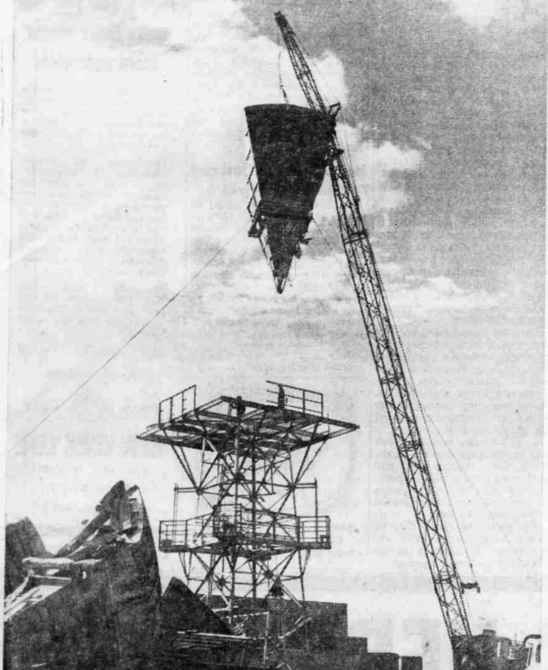
ANTENNAS HOISTED — Microwave antennas, weighing two tons each, were hoisted into position by mobile crane last week at Pacific Telephone and Telegraph company's new microwave relay stations at Baldy mountain (shown above) and Siskiyou summit. The scoop-shaped antennas, each 22-feet long, were put in place on 37-foot structural steel towers. The relay stations will provide a link between Sacramento to Portland for television programs for three networks and telephone conversations. Both TV programs and conversations are carried through coaxial cable now. The stations are expected to be in operation next August, according to PT&T officials. —(Pacific Telephone photo.)
