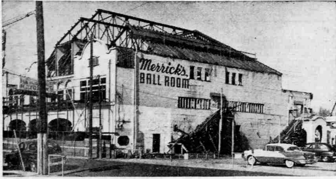
OLD 'NAT' COMING DOWN —One of Medford's best-known landmark buildings, the old "Natorium," is coming down. The picture above shows the progress made so far by the wrecking crews. The building, known in more recent years as Merrick's Ball Room, has housed a wide variety of activities during its long history, including grand opera, swimming, shooting in a basement range, boxing and wrestling, plays, and dances. Tentative plans are being made for construction of a 40-unit downtown motel, with restaurant and swimming pool, on the site, which is a block north of Main st. on Riverside ave. —(Brainard photo)
