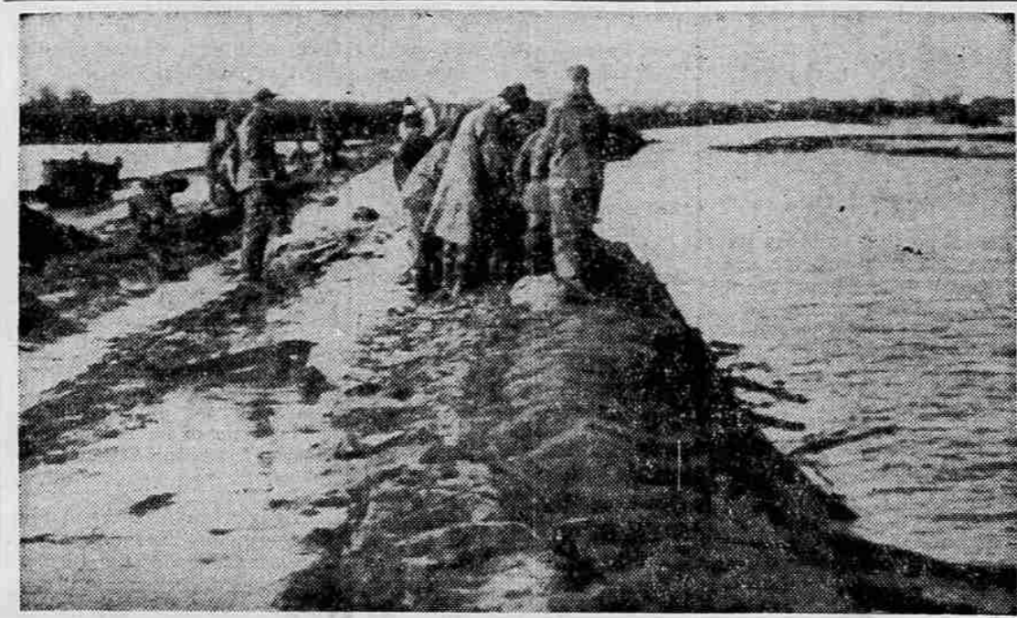
BATTLE RAMPAGING RIVER —Troops from Camp Beale labor to bolster weakened section of the levee along the Feather River at Yuba City, Cal., in an effort to prevent a repetition of the Christmas week disaster which cost the lives of 33 persons when the city flooded. Engineers called the situation critical.
