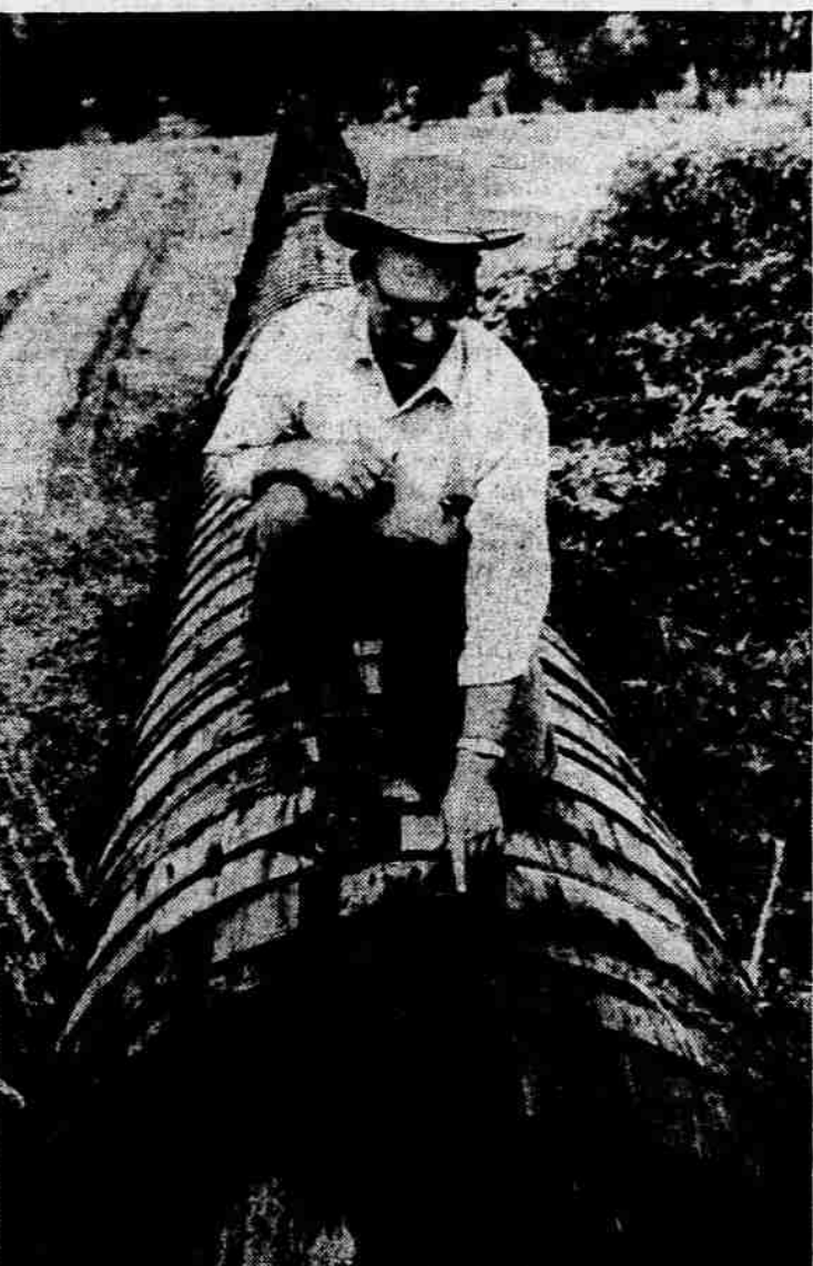
LEAKS IN OLD SIPHON — Jack Hoffhuhr, manager of the MID, is shown above pointing to one of the many leaks in the siphons used by the irrigation districts to get water to the valley floor. It is proposed to replace these slowly rotting, antiquated structures with concrete siphons. It is believed that the savings in maintenance costs alone will permit repayments on a contract with the government to be made without increasing water assessments. If the system failed at any of its weak points, it could be up to 30 days before service could be restored, which might well mean a total crop loss in the districts.
