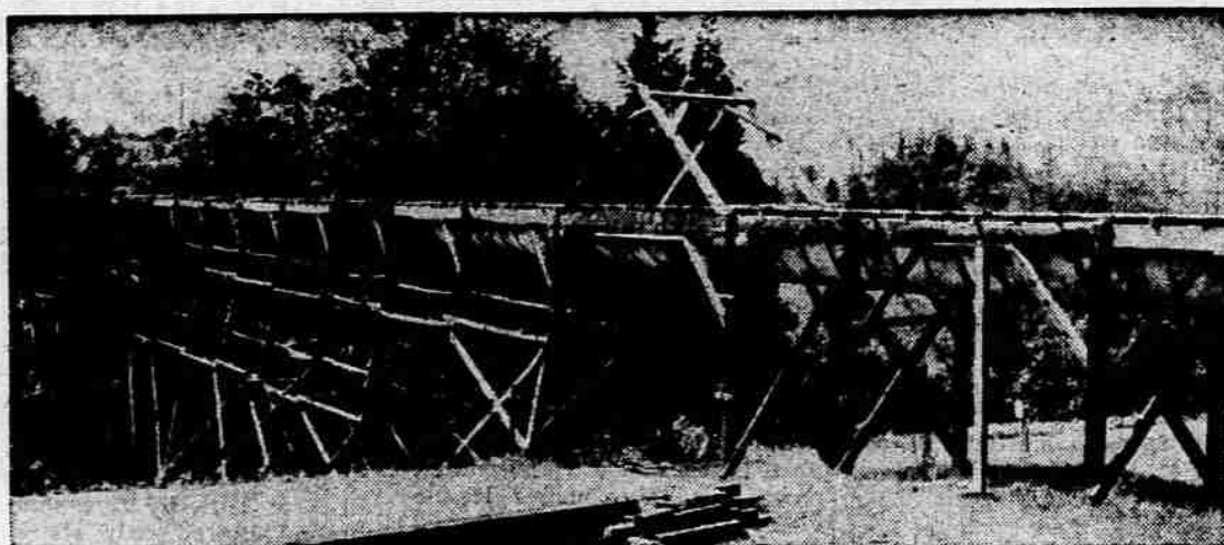
OLD FLUME CARRIES CANAL — One of the chief reasons that rehabilitation is being sought for the canal system of the Medford and Rogue River Valley Irrigation districts is the old structures, built more than 30 years ago of untreated wood, which are now in
