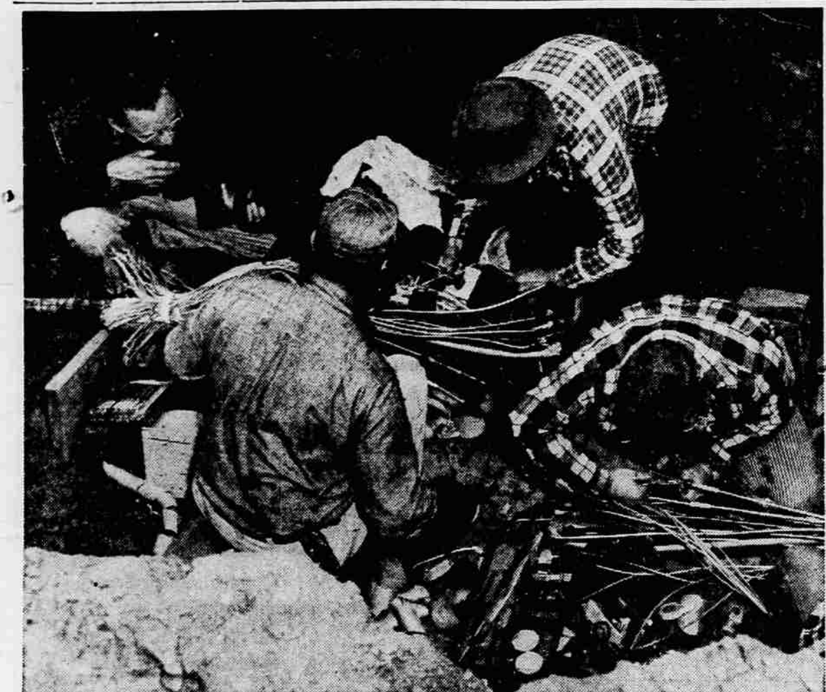
QUITE A JOB —Telephone company repairmen are shown above involved in the complexities of repairing a coaxial cable which was cut in two by a ditching machine north of Medford yesterday morning. The mishap halted the flow of both United Press and Associated Press news to The Mail Tribune, Ashland Tidings and Grants Pass Courier, as well as to the radio and television stations, and in addition interrupted
