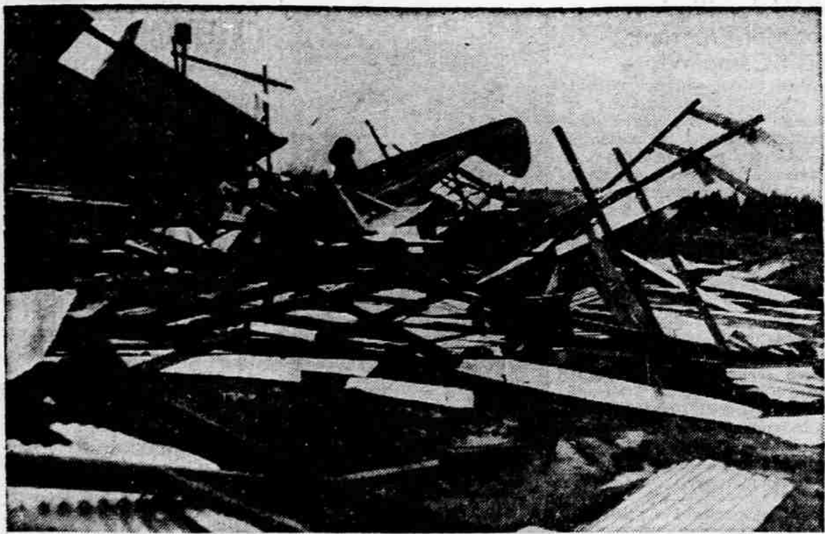
WINDS HIT OREGON —Winds up to 75 m.p.h. tore these steel hangers apart and wrecked five planes at Trohs Air Park in Portland, Ore. Sixteen other planes came through undamaged when the hangers they were housed in blew apart. Damage was estimated at $50,000.
