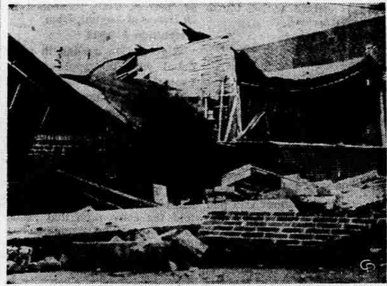
RIPPING STRUCTURE APART , gas explosion at Allen, Okla., school injures 34 children, two seriously. Police official said it was "near miracle" no one was killed. (International Soundphoto)
