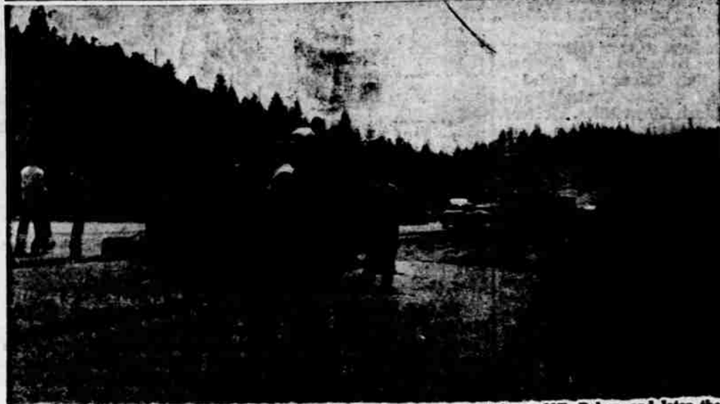
Above, in 1926, they "spread the hot stuff" the hard way on Highway 99E. Below, and later they "laid it along" evenly and easily—more machines, fewer men; four times the progress. (State Highway Commission Photos).
