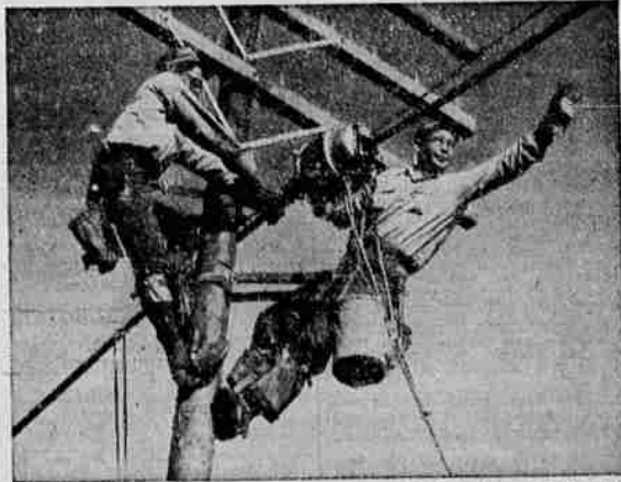
No one can guess the importance of the calls which will flow through the cable these linemen are installing.
