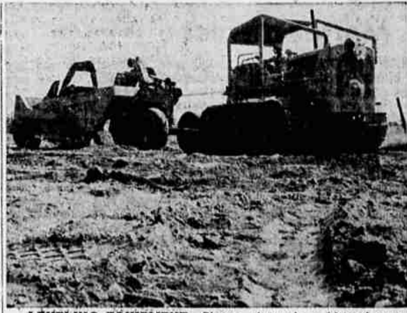
LEVELING EQUIPMENT —Shown above is a 10-yard carry-all being pulled by a caterpillar from the Tru-Mix Equipment company which contracted the leveling job under the conservation practice of preparing land for irrigation, described in the accompanying article. The carry-all scoops the dirt off the high points and dumps it over the lower places which in the accompanying picture were covered with rocks. This implement is followed in the leveling procedure by a "ripper" which evens up the ground consistency so it will all settle at the same level rather than unevenly at the soft spots. The ground is then land-graded and ditched before seeding to permanent pasture.
