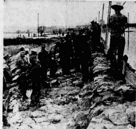
DAY OF CRISIS —Today is the "day of crisis" in the Missouri river flood picture, according to Army engineers. Shown above are the levees at Council Bluffs, Ia., as workers, standing in muddy water, pass material to bolster the walls against the "tremendous pressure" of the swollen river, which forces water through the levees. —(International)
