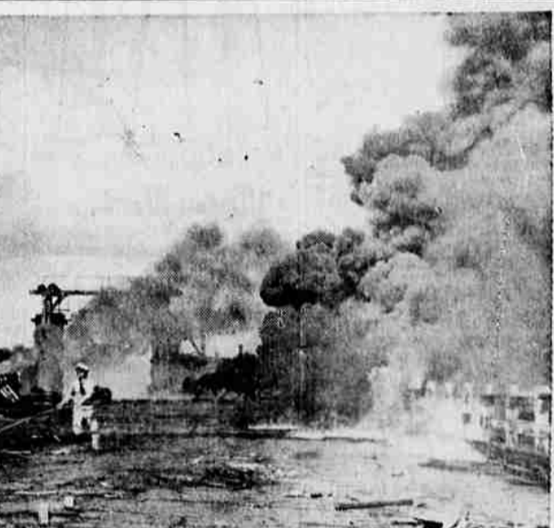
BURNING THE PAST—The past goes up in smoke as Navy Warrant Officer Roland D. Foster sets fire to an abandoned ferry mole in Alameda, Calif. The mole was destroyed because rotting piers, driven in the last century, have been breaking off and floating into the path of seaplanes landing and taking off at the Alameda Naval Air Station.
