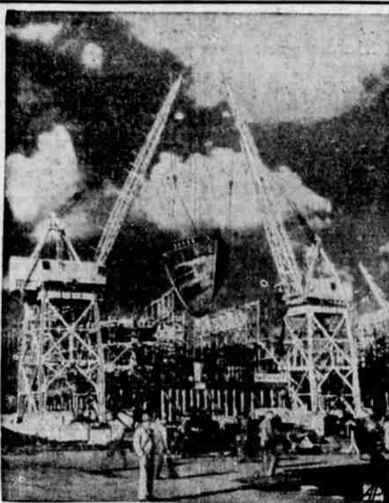
The entire forepeak section of a Liberty ship's bow, made of pre-fabricated material, was hoisted into place on the way at the California Shipbuilding Corporation's yards at Wilmington, Calif., to make for greater speed in shipbuilding. Pre-fabrication of large sections of the 352 Liberty ships now under construction or contracted for makes for faster production.
