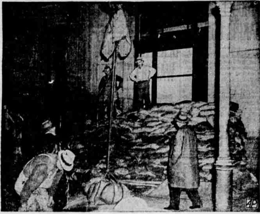
Workmen were busy in San Francisco raising a barricade of 3,000 sandbags around the long distance building of the telephone company as a protection against possible bomb damage.
