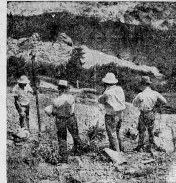
FIRST TEST BORINGS at site of Shasta dam, immense unit of Central valley project, were made here. In background is Sacramento river and just below hill on which, men stand is railroad for which temporary diversion tunnel will be built.
