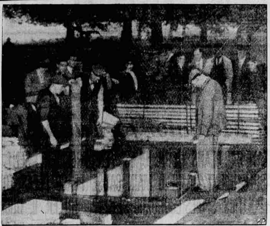
While the anti-aircraft and coast defense units of Britain's territorial army were called out as Europe's eleventh hour of peace or war approached, London pushed its preparations for the worst. This picture, sent by radio to New York, shows an air-raid dugout being constructed in Hyde park.
