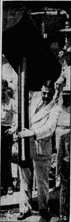
SLUDGE AND SLUDGE. Driving the first pile into Mississippi mud, Governor Leche of Louisiana uses a huge sledge to start a $10,000,000 bridge.
