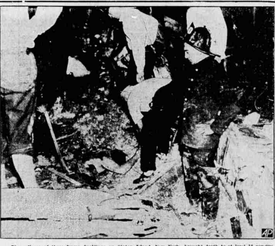
The collapse of three frame dwellings on Staten Island, New York, brought death to at least 18 persons. Police and firemen are shown searching the ruins. Heavy rains were said to have been the cause of collapse.
