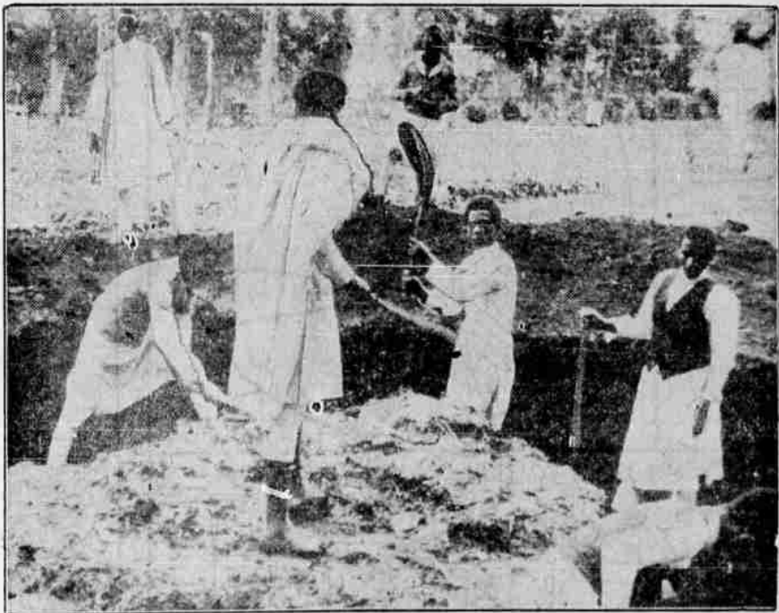
Convict laborers have been put to work in Addis Ababa, capital of Ethiopia, digging trenches for use in the city's defense should Italian troops attempt to occupy it. (Associated Press-Paramount News Photo)
