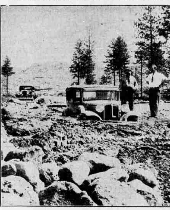
Scores worked feverishly repairing 1000 feet of Southern Pacific railroad tracks and the Weed-Klamath Falls highway in northern California, near Black Butte, when they were washed out by cloudbursts. Thousands of tons of boulders, trees, dirt and water were brought down Whitney glacier to halt traffic. One of the trapped cars is shown. (Associated Press Photo.)
