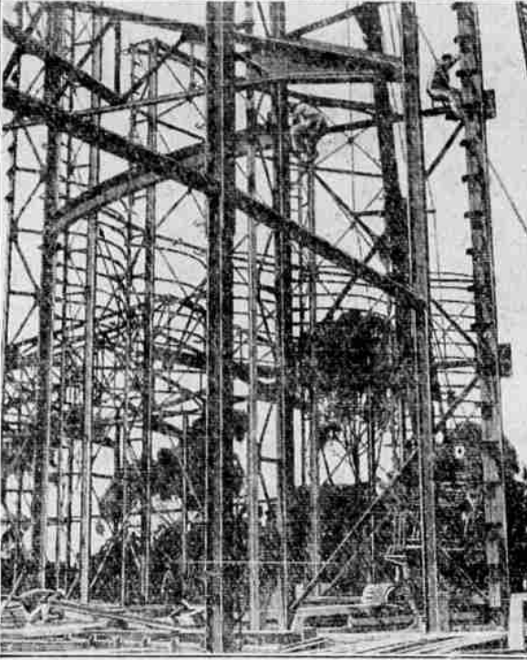
With nearly 100 per cent of the steel work erected, contractors promise completion within the next few days of the steel work for the Ford Motor Company's exhibit palace at the California Pacific International exposition, San Diego, opening May 29. Then pouring of concrete for the great circular exhibit building will get under way.
