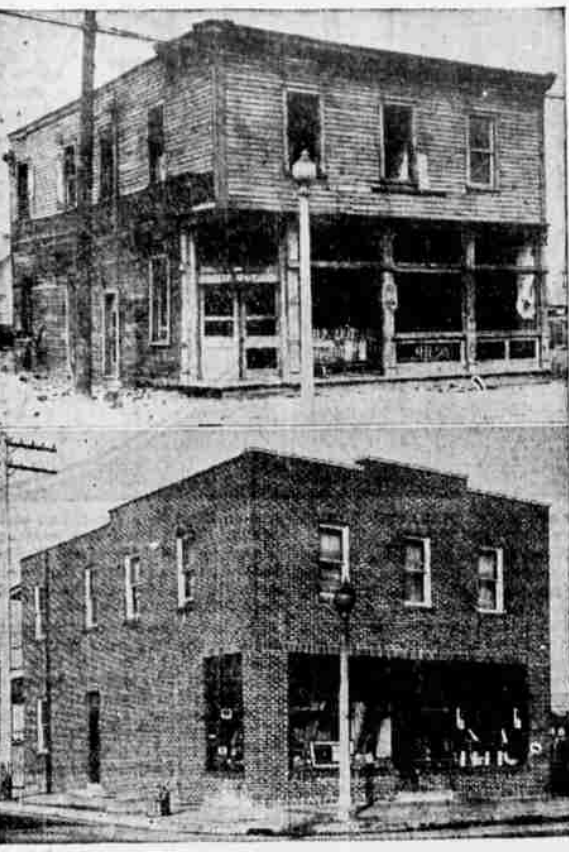
The building pictured in the upper illustration apparently was beyond repair. An examination, however, revealed a sturdy frame, so modernizers converted it into the attractive store shown below.
