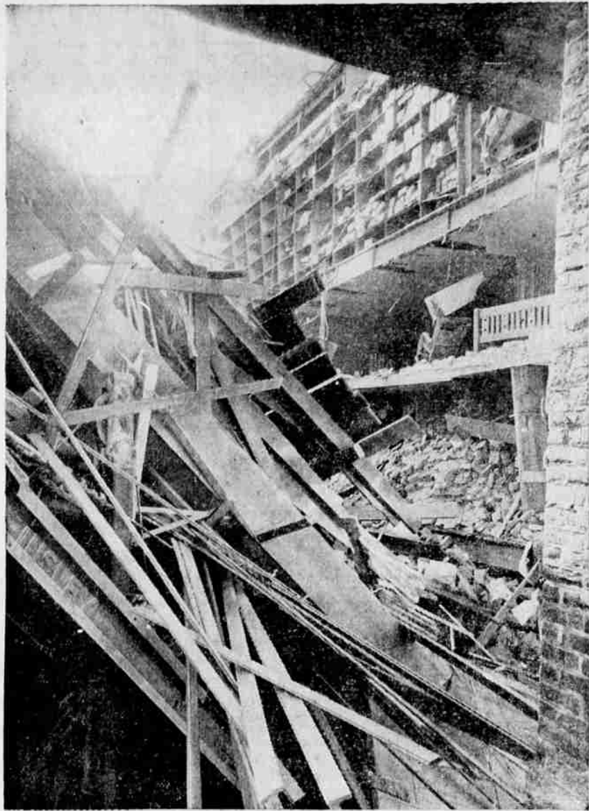
Workmen have nearly cleared away the tons of debris that half-filled the newly-excavated basement of the Scott Davis building, formerly the Hutchison Mercantile Co., when an adjoining wall of Mann's Department store caved in Saturday night, followed soon after by a large section of the ceiling and roof. After closing for three days to batten the side of the building laid bare when the brick wall crumbled and to clear away billows of dust, Mann's Department store reopened. Debris from the cave-in knocked out part of the east wall of the stock room of Swann's Gift shop, which is now also nearly repaired and braced against further cave-in. A brick wall left standing along the alley will be completely torn down before workmen begin reconstruction of the buildings, which, although the east wall of Mann's was to have been removed anyway, were damaged to an estimated extent of $50,000.
