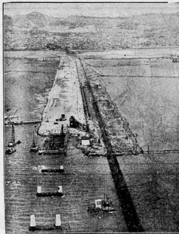
Millions of cubic yards of sand dredged from San Francisco bay bottom are going into the fill of the Oakland or eastbay approach of the San Francisco-Oakland bridge. This aerial view shows the bridge foundation piles in the foreground and the fill to the left of the railroad tracks. (Associated Press Photo)
