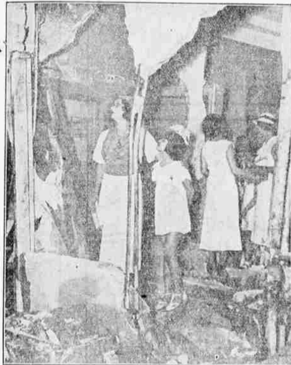
Devastation wrought in the recent battle of the Hotel Nacional in Havana now may be seen by visitors. Sight-seers are shown inspecting damage caused by one shell which pierced three walls and exploded 40 feet inside the building. (Associated Press Photo)
