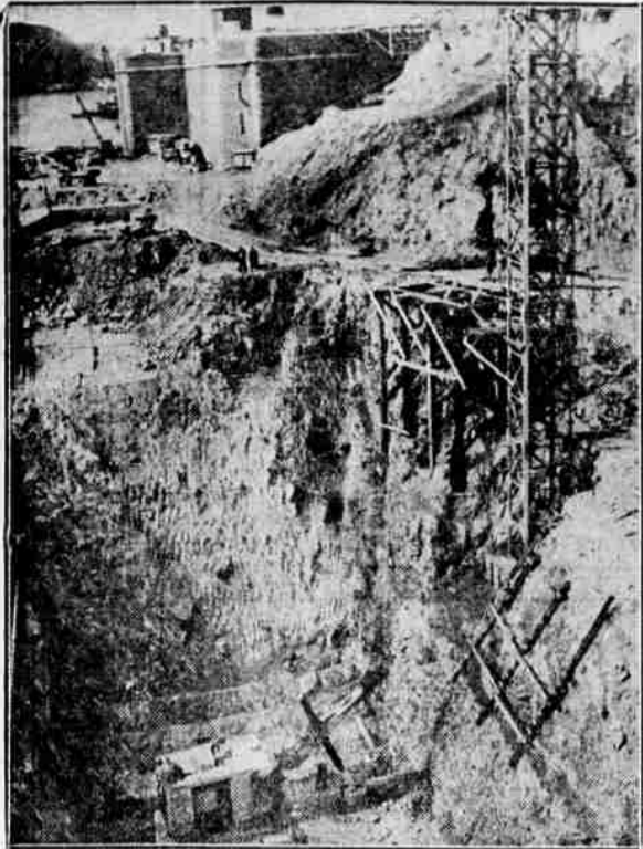
This excavation will be filled with 64,000 tons of concrete and will be one of four "anchors" of the same size for the Golden Gate bridge crossing the entrance of the San Francisco bay. This hole is on the San Francisco side and the Golden Gate can be seen in the background. (Associated Press Photo)
