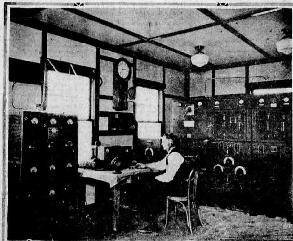
In interior of KCX; in front of Mr. Martin is the receiving sets and microphone. In the foreground is the short wave transmitter used for code communication between airway stations. Large panels back of Mr. Martin are those of voice transmitter.
