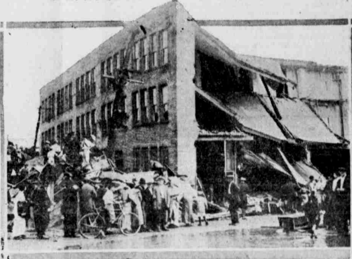
Ruins of what once was a wagon manufacturing plant. Two people were killed at this spot. Photo shows crowd searching for other bodies.
