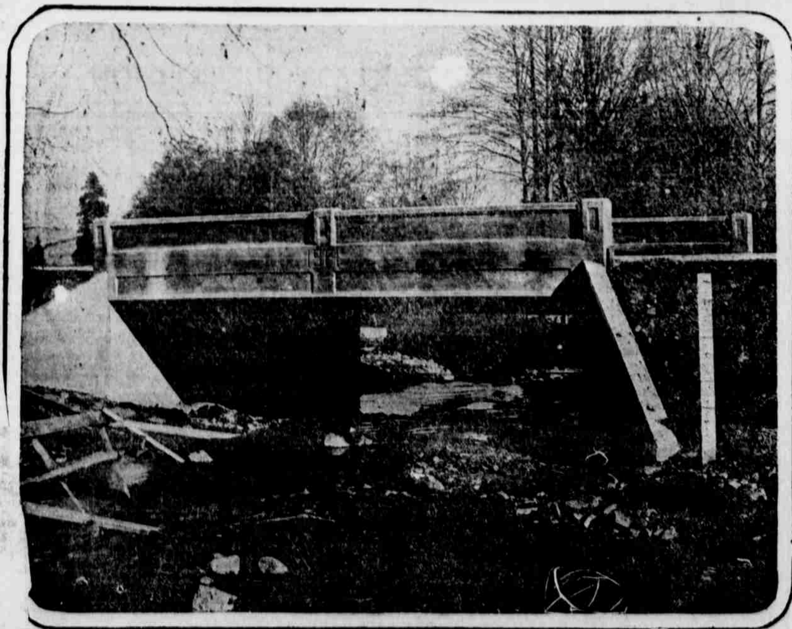
Type of Concrete Bridge Erected Along Pacific Highway in Jackson County.—Photos by E. D. Weston, Medford.
