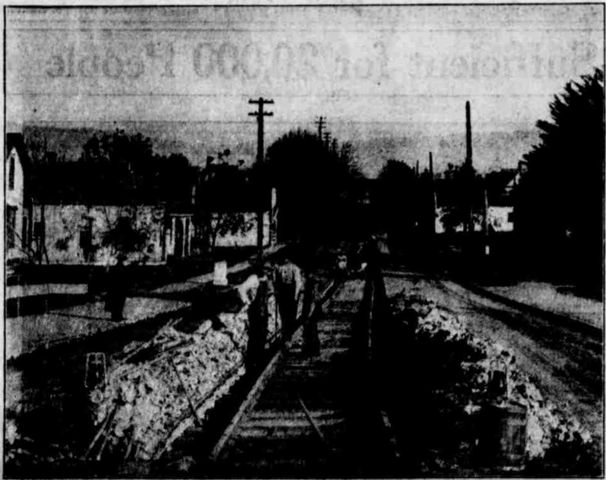
Construction crew at work on East Main street on Southern Oregon Traction Company line, franchise for which was granted Spencer S. Bulls of Olean, N. Y., last May. Line will be in operation in March and will eventually be extended throughout the valley.
