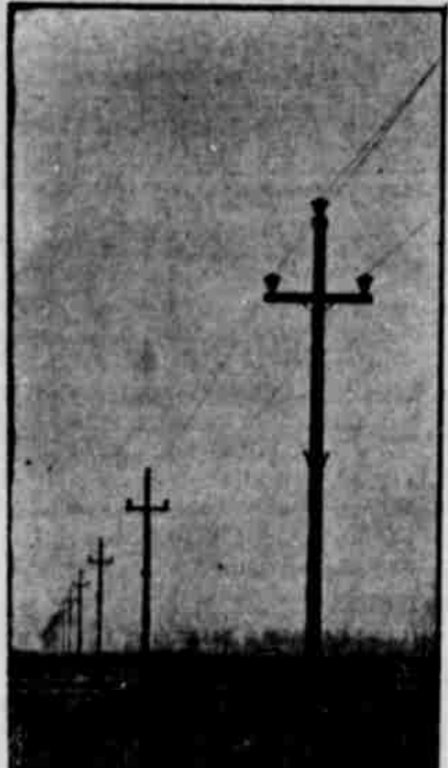
Prospect Pole Line
