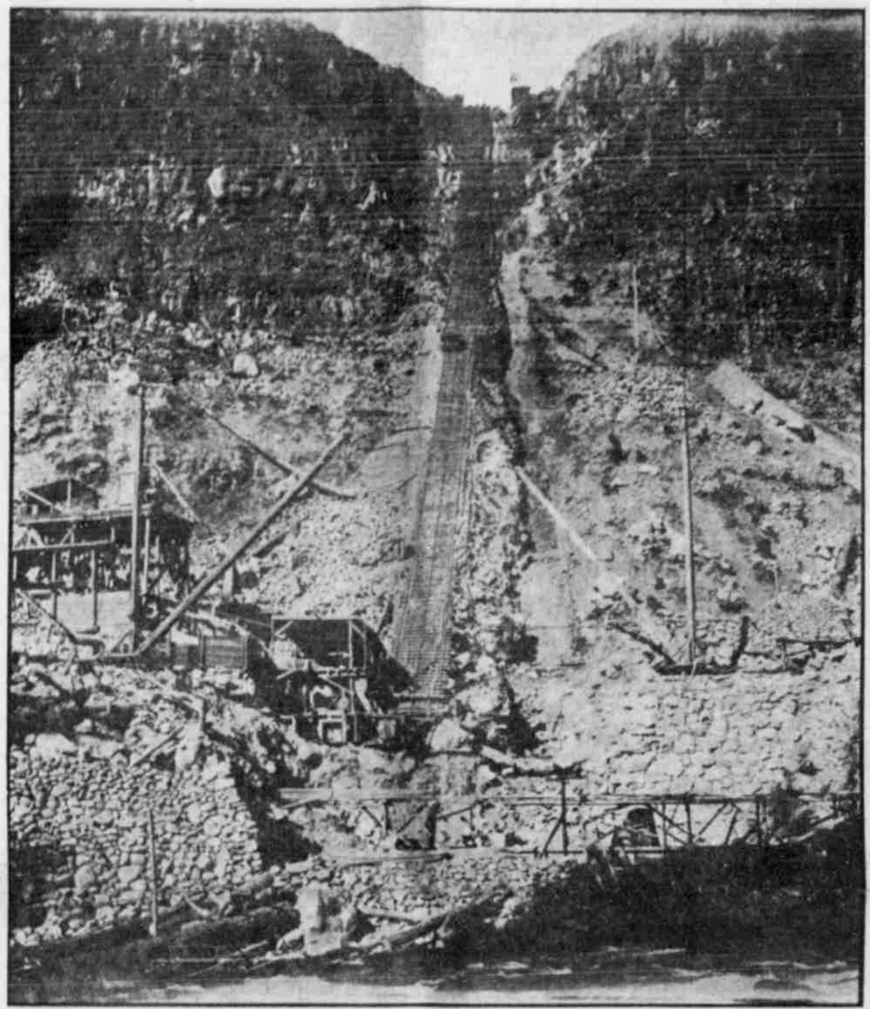
This shows construction work in progress on the new power plant at Prospect which is now ready for business.
