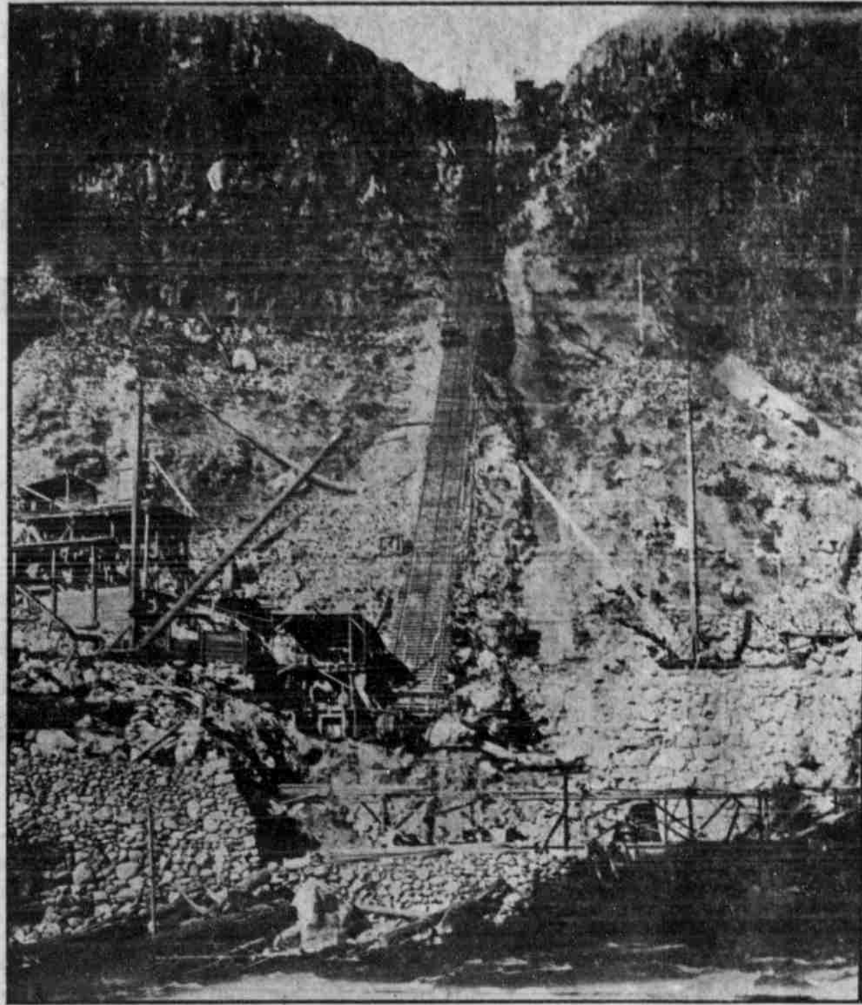
Site of Power House and Excavation for Drop Pipe—Great Fall Is Secured.
