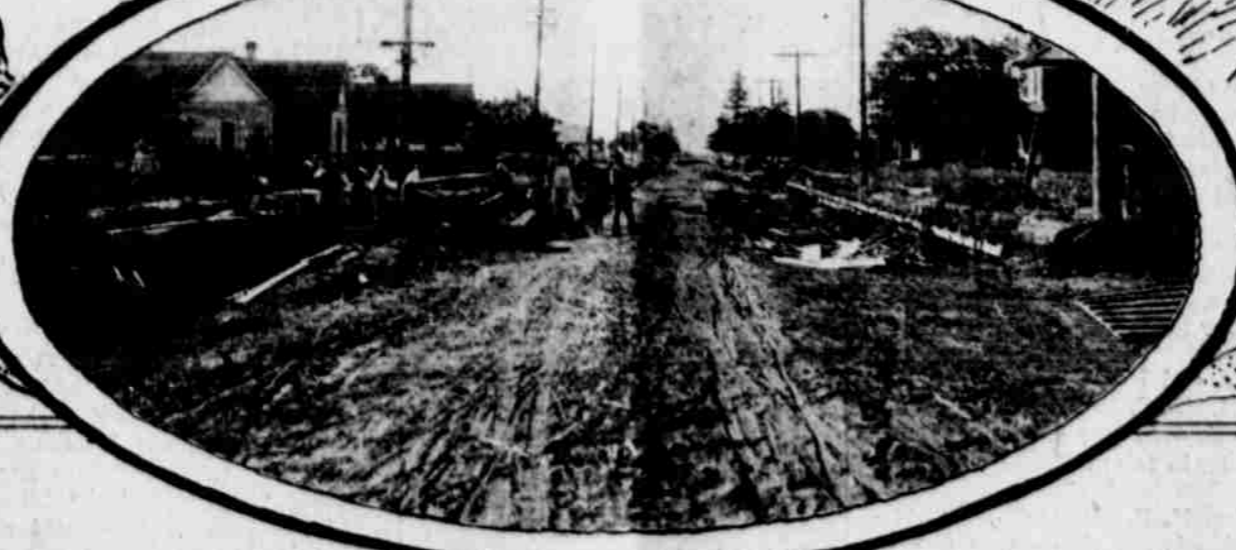
Upper Line Shows Grading Camp and Paving Plant; Second Line, Concrete Base Gang and a Gang Laying Surface, Third Line Shows the Concrete Mixer and Grader, the Fifth the Curb and Gutter Gang of the Clark & Henry Construction Company
