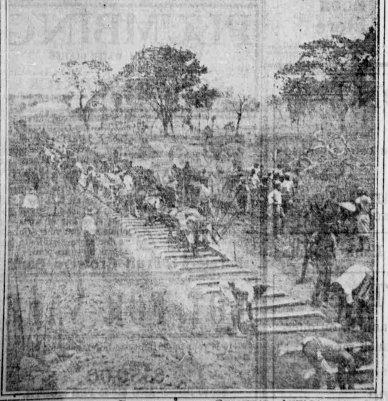
Native are here putting down sleepers on the Katanga railway, approaching the star of the Congo mine. Metal sleepers are used in the construction of the line instead of wooden ones as is usually the case. The reason is partly because metal sleepers are more durable, but chiefly on account of the swarms of ants which abound in the Congo and would quickly make short work of wooden sleepers.
