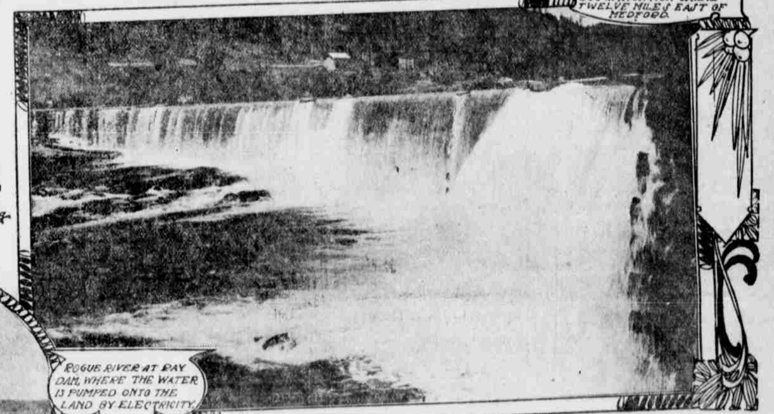
COMPLETED SECTION OF ROGUE RIVER VALLEY CANAL CO'S IRRIGATION CANAL TWELVE MILES EAST OF MEDFORD
