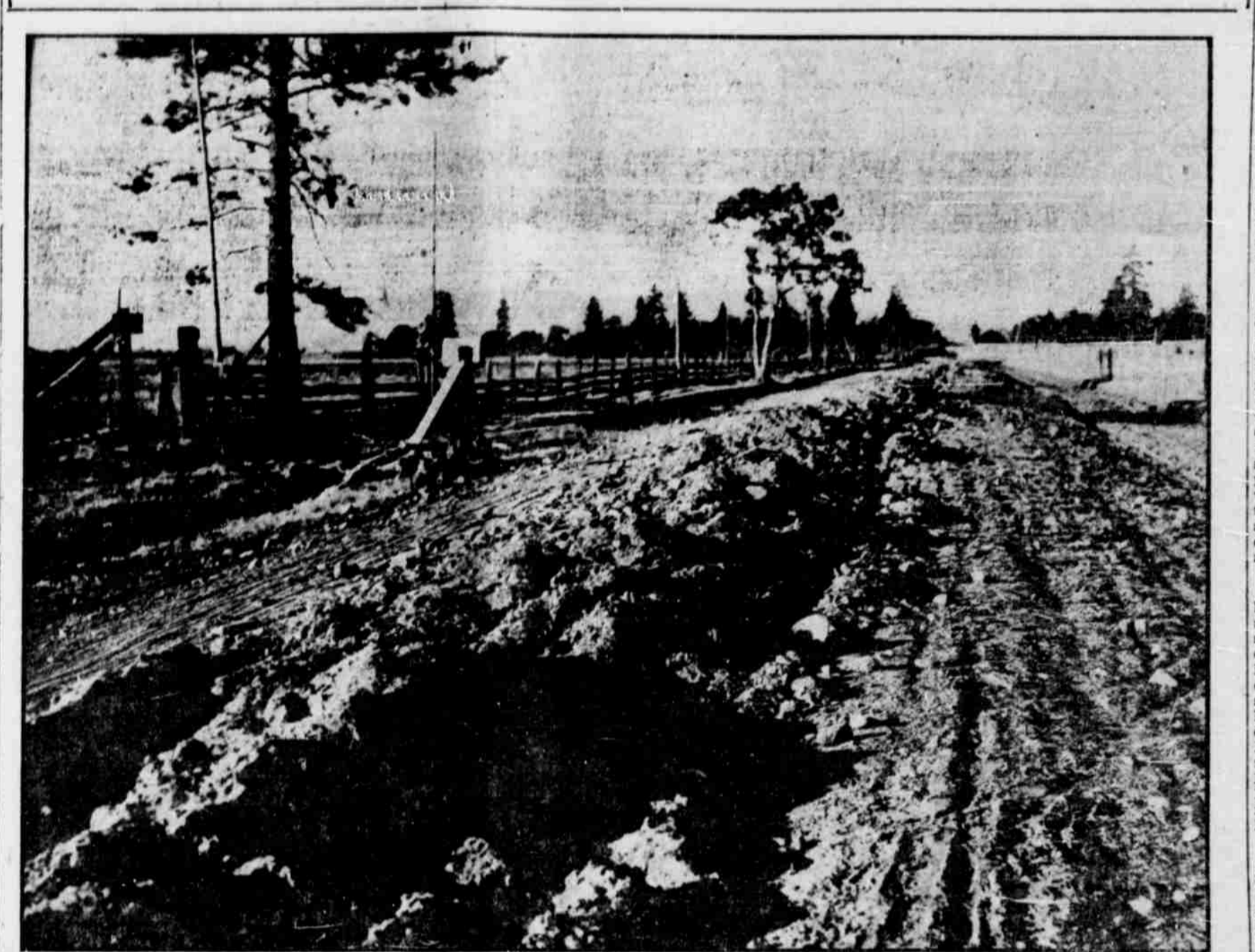
Photo of a county highway constructed by Joshua Patterson, for eight years past county commissioner, who, being defeated in the direct primaries for republican nomination, seeks re-election as an independent. This shows methods of construction; gravel and cobblestones being dumped three feet high in center and left all summer for the traveling public to level off when wet weather forces travel out of the gutter on either side. No attempt is made to roll or smooth off.
