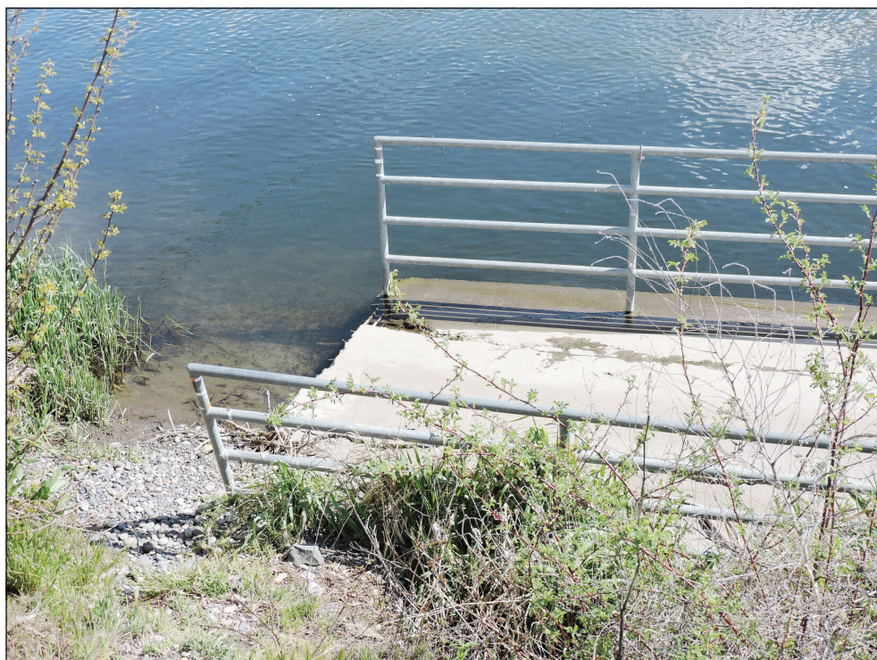
A broken section of a destroyed Umatilla River footbridge sits on the shore on April 14, 2022. Erick Peterson/Hermiston Herald
