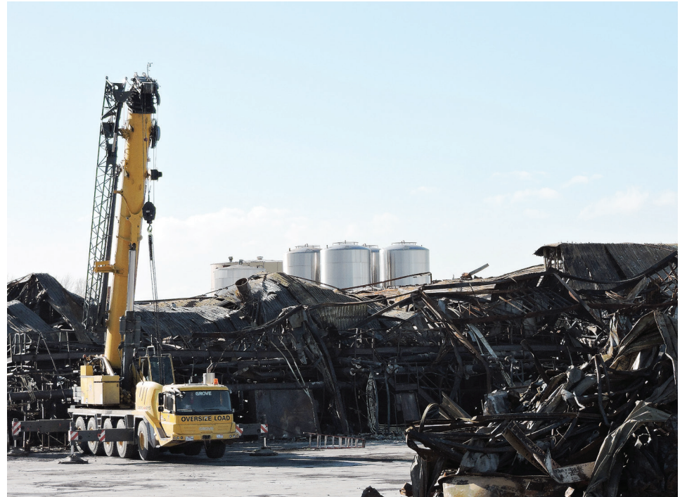
Equipment was in place to remove sections of debris from the destroyed Shearer's Foods plant in Hermiston on Monday, April 4, 2022.
