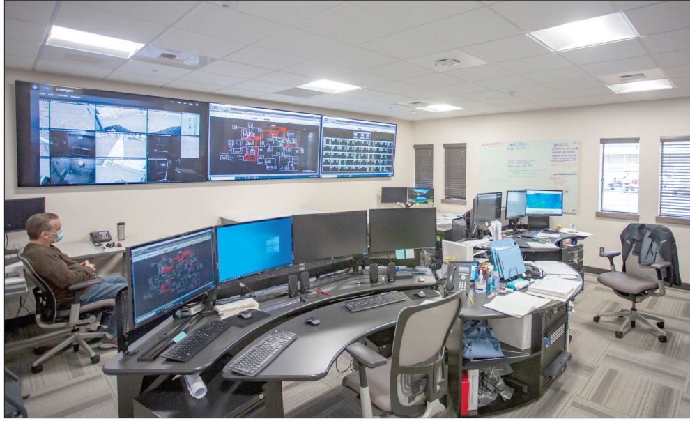
A control room at Umatilla Electric Cooperative in Hermiston oversees operations and systems across the cooperative's coverage area.
