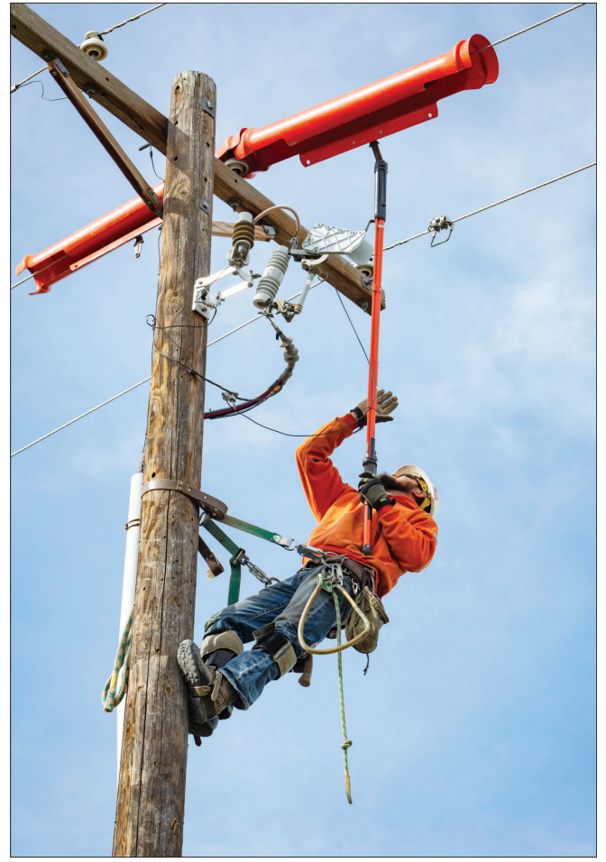
Matt Ellis, a lineman with Umatilla Electric Cooperative, positions equipment atop a utility pole in Hermiston on Wednesday, April 7, 2021.
