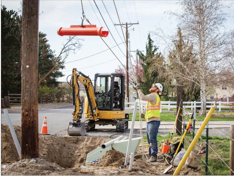
Nick Hardie uses a rope to raise equipment up to fellow lineman Matt Ellis, while working on a utility pole in Hermiston on Wednesday, April 7, 2021.
