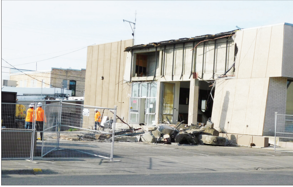
Contractors begin tearing down the former Hermiston City Hall on the morning of Wednesday, March 17, 2021. The building will be replaced with a larger facility in the same location.
