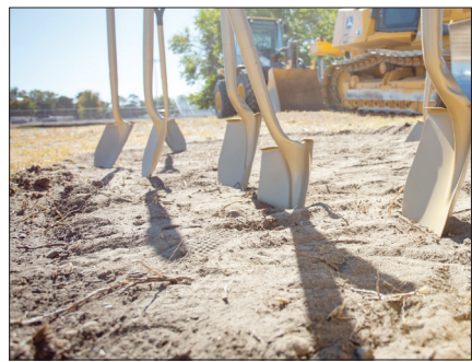
Shovels sit in the dirt at the site of Hermiston High School's new softball complex during its groundbreaking ceremony on Tuesday, Sept. 29, 2020.
