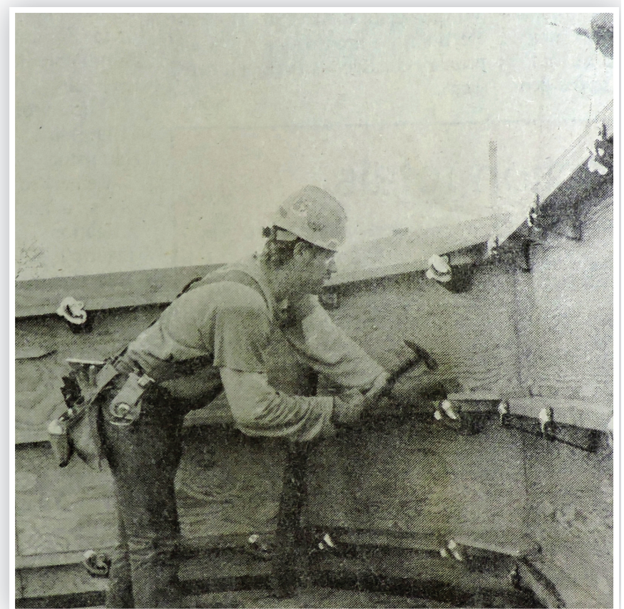
Jim Hudson of Hermiston works on constructing what would become Sandstone Middle School in 1994.
